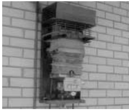
Lack on servicing has resulted in a melt down of this water heater's heat exchanger
