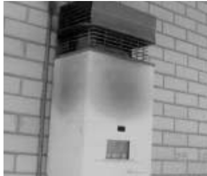
Radiant heat from the melt down has damaged the water heater's cover
