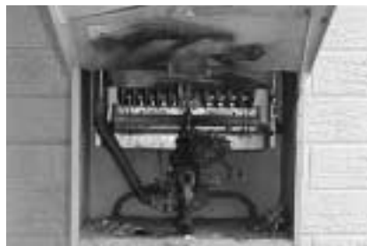
A different water heater – a melt down has destroyed the appliance
