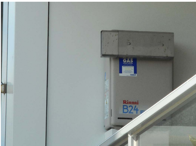
Fan assisted water heater with sideways draft diverter
