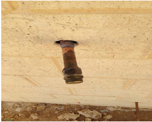
Compliant temporary termination
