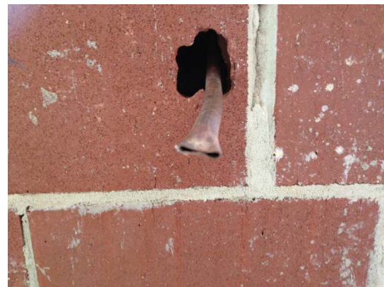
Non-compliant temporary termination
