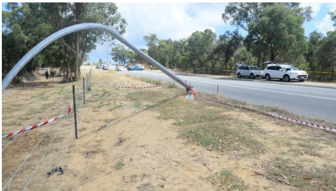
Damaged metallic streetlight pole
