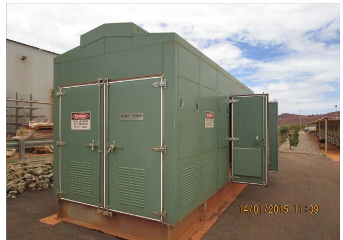
Kiosk pad mounted substation located outside the warehouse
