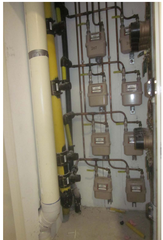
Non-compliant PE riser prior to replacement
