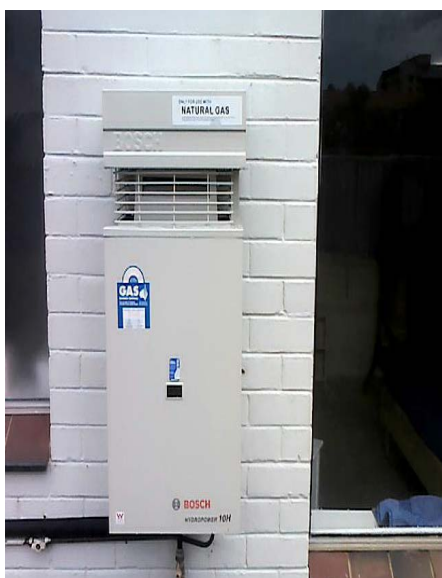
Non-compliant gas hot water system installed too close to window
