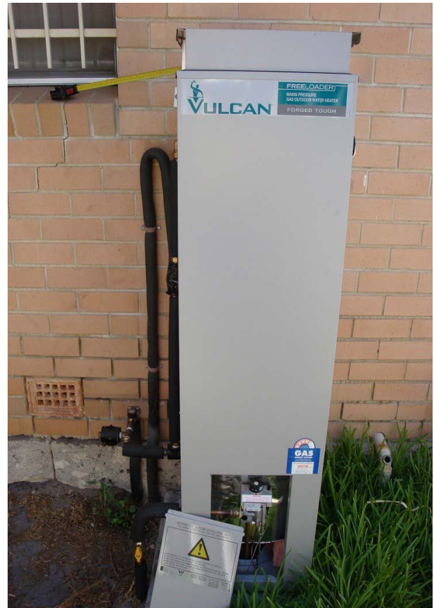
Non-compliant gas hot water system installed too close to window
