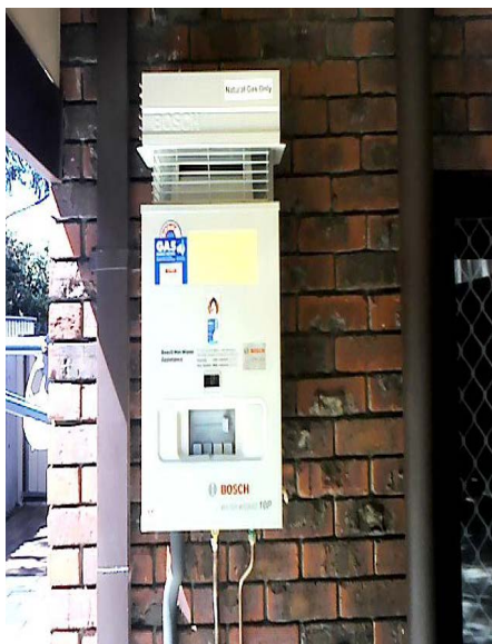
Non-compliant gas hot water system installed too close to return wall and downpipe
