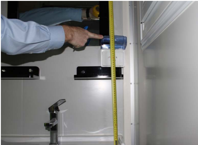
Socket outlet installed in a wet area
