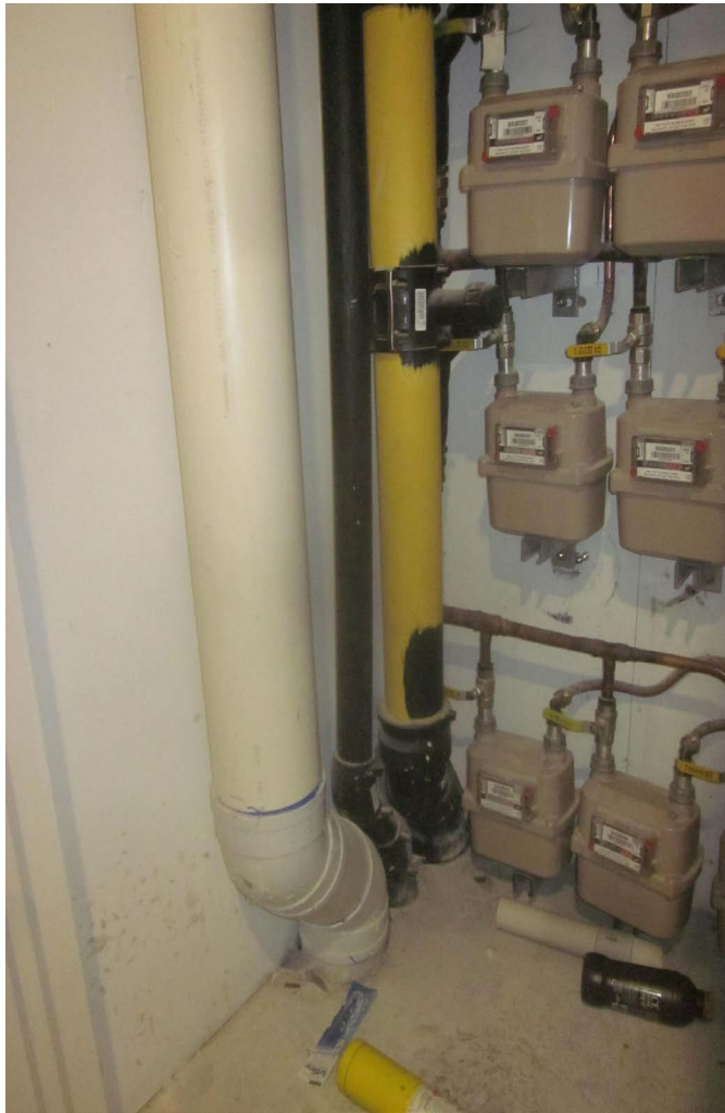
Non-compliant PE riser prior to replacement
