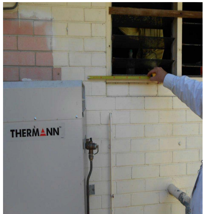
Non-compliant gas hot water system installed too close to window
