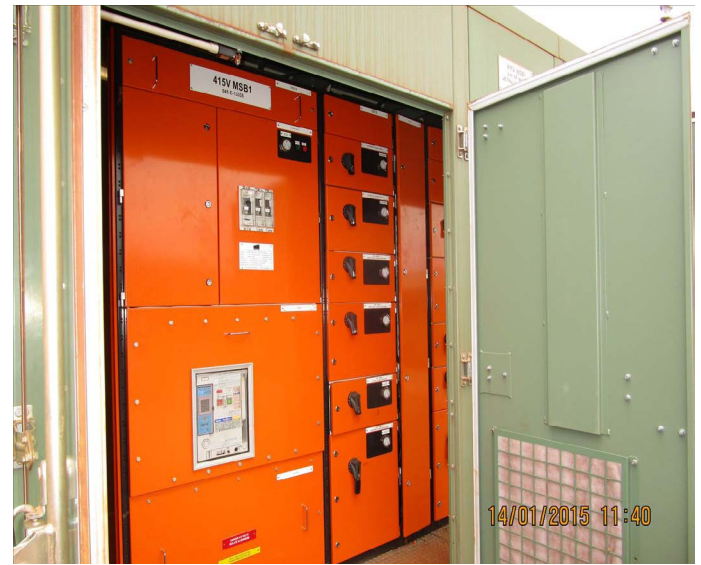
Distribution boards located within the warehouse
