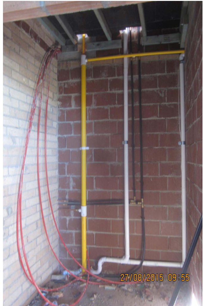
Non-compliant UPVC pipe installed in wall cavity
