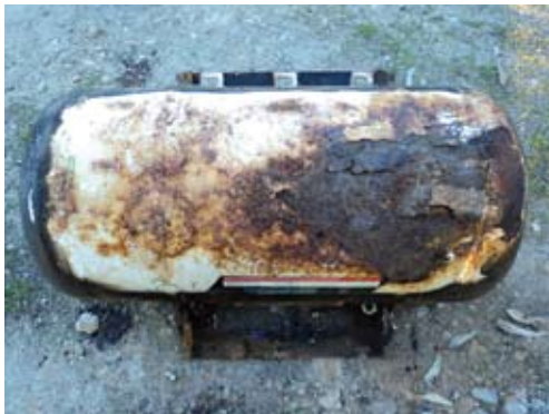
Showing the underneath of the LP Gas fuel container with guard removed.
