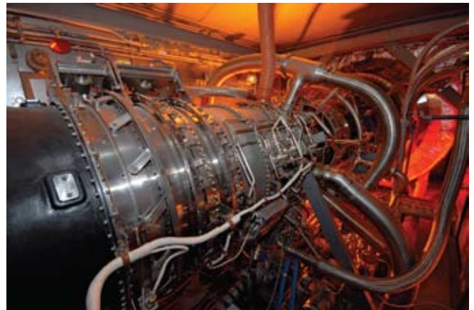
Kwinana Swift Power Station gas turbines
