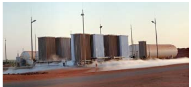
Broome LNG Fuel Storage Facility
