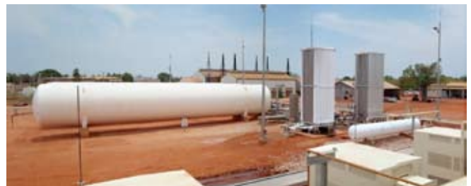
Derby power station (12MW)
