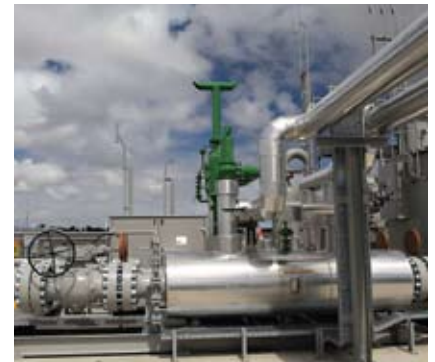
Neerabup Power station Gas yard
