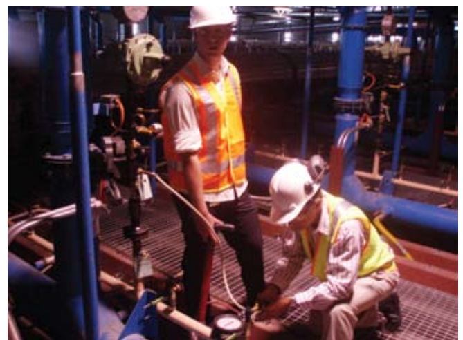
Conducting a pressure test on BGC's new brick kiln burner gas trains. Pictured (from left): Alex Hayes and Kim Martin
